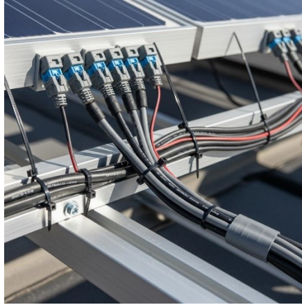
Figure 4.5: Connectors and DC cables
