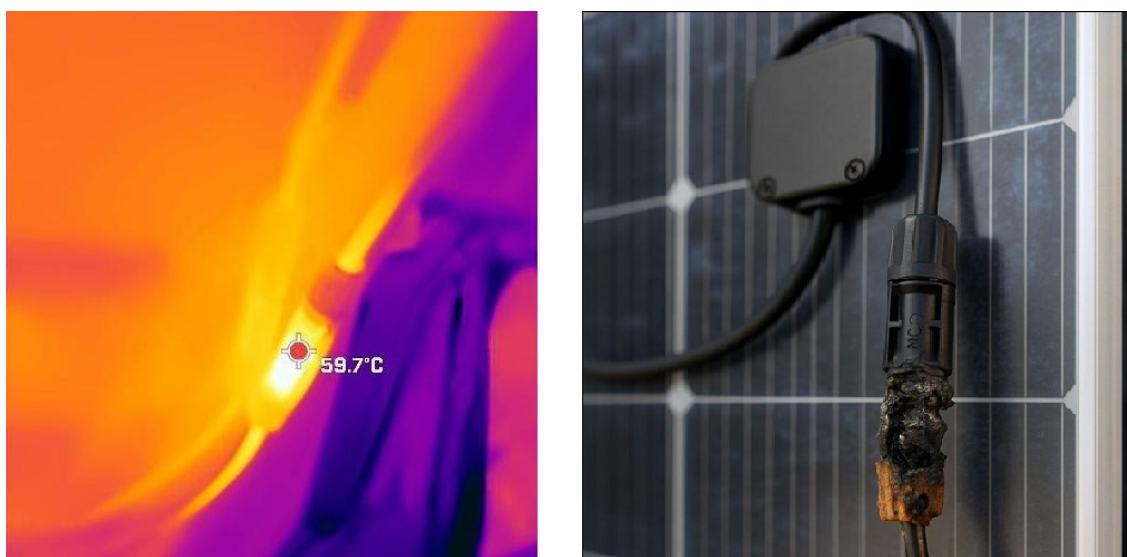
Figure 3.15: Overheated PV connector
